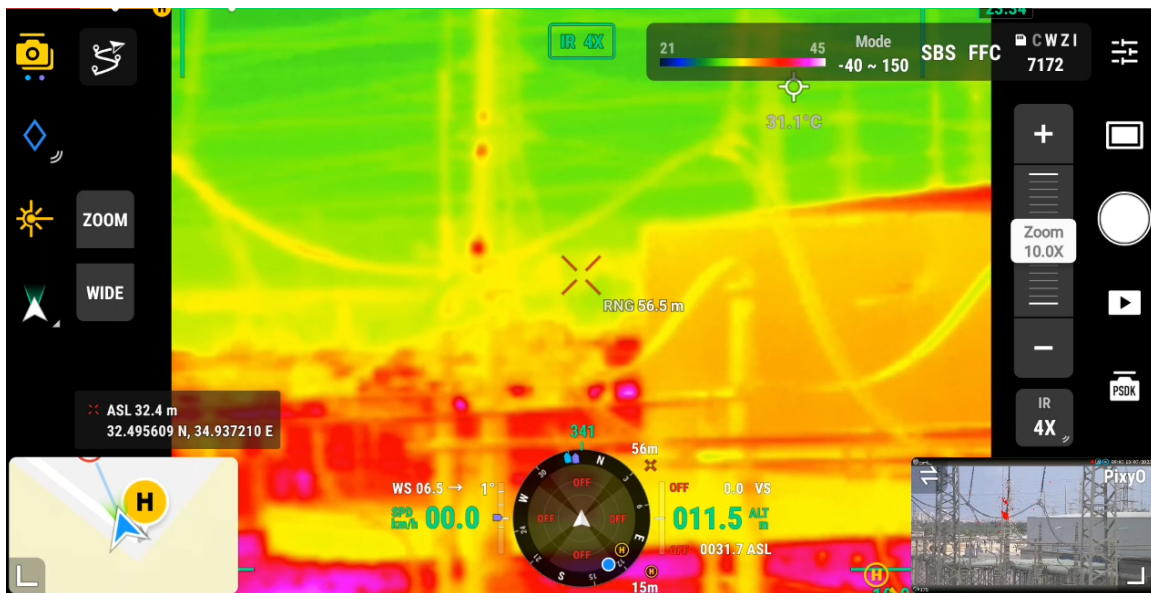
Hotspots and corona discharges detected on a high voltage bushing
