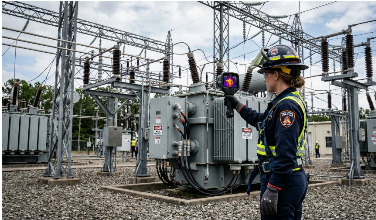
Substation inspection with a thermal camera
