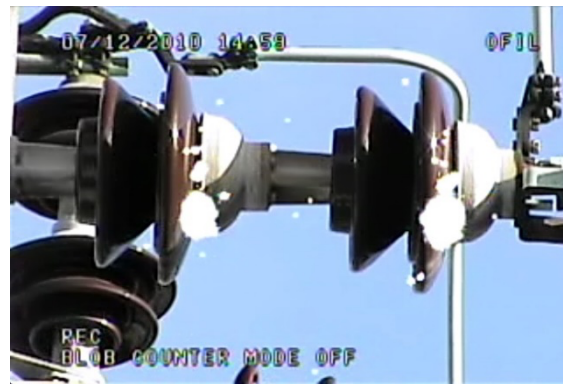
UV image: two spots of corona discharge detected
