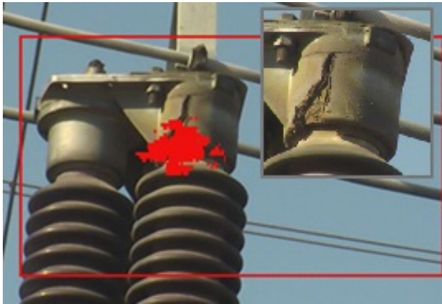
Corona discharge activity on HV insulator detected using a UV camera
