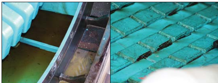
Subjected to oil (above left), wedges, side packing, and top ripple springs softened and loosen. In an oil-saturated environment, loose wedges will produce a greasy-type byproduct (above, right).
